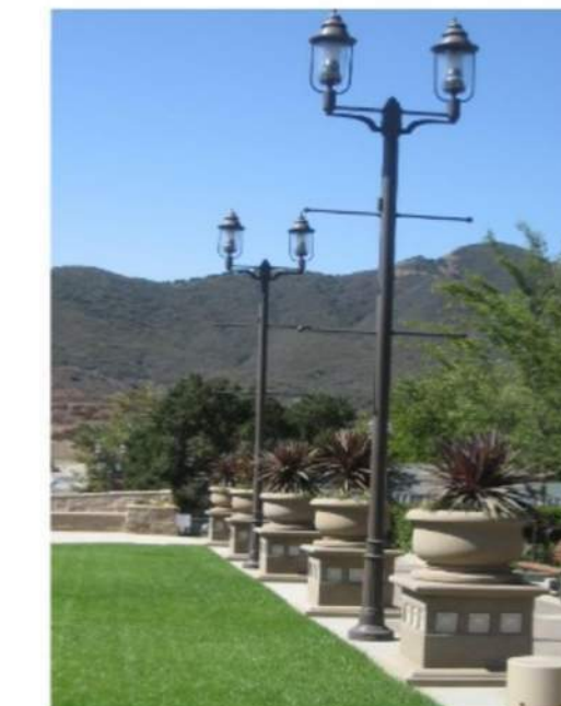
Figure V-135 a,b: Examples of decorative double posted lantern style light fixtures in Old Town.
